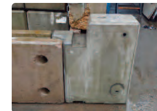
VCB End Section
